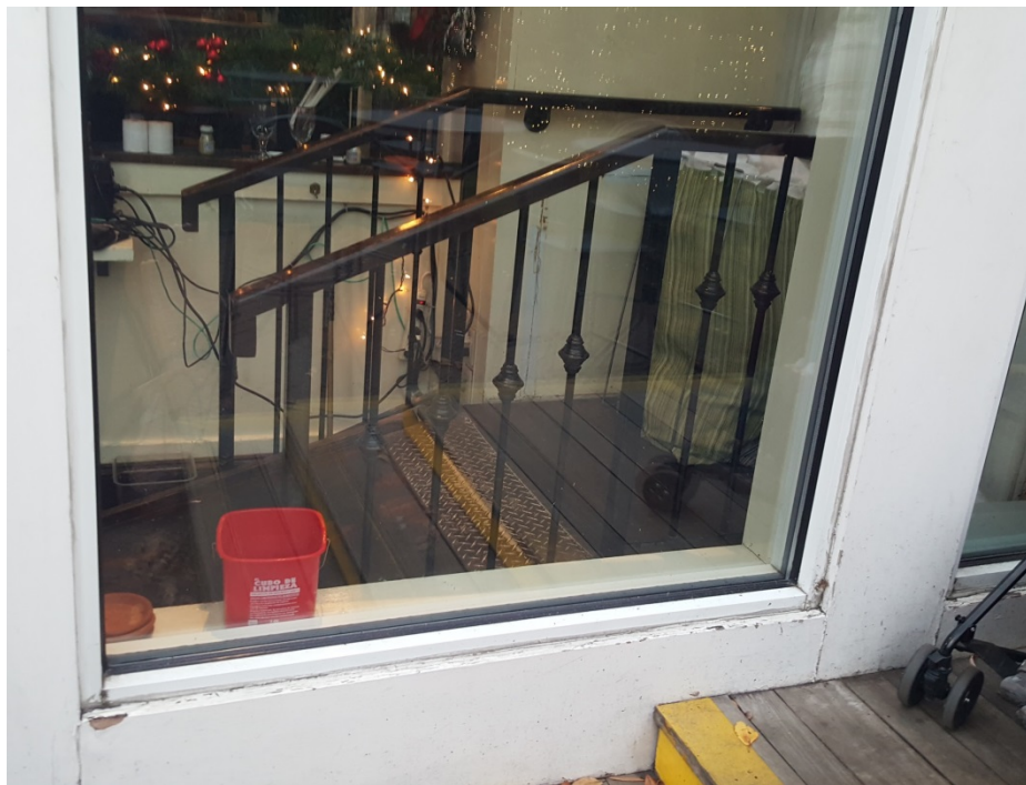
Figure 2 - Photograph of Metal Ramp; visible are steps from Middle Level to Lower Dining Area and equipment blocking access to the ramp, itself of a non-ADA-compliant style. Taken Dec. 26, 2015.
