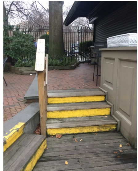
Figure 5 - Photograph of Outdoor Bar showing close up steps up to it from Brick Patio and Boardwalk. Taken Dec. 26, 2015.
